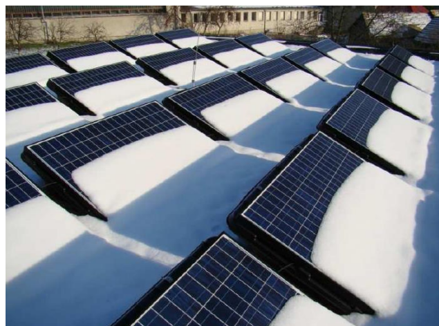
Figure 5. Solar panels installed on roof of the model house, partially covered by snow
